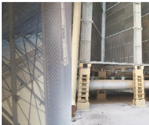
Fig. 2. Delta view and tube arrangement in the dry cooling tower
