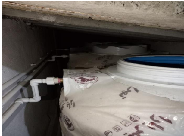
Fig. 6. An example of non-visitable polyethylene cisterns
