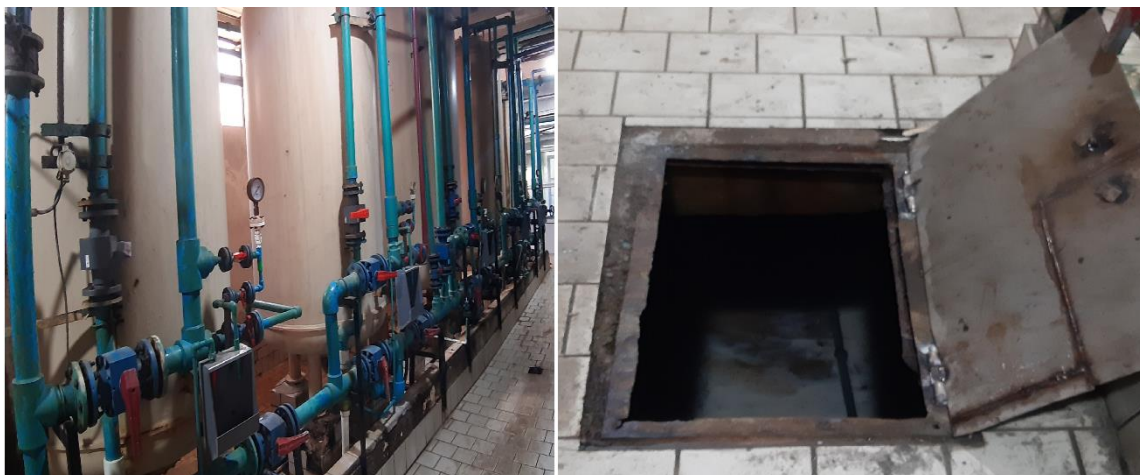
Fig. 4. The image of cationic, anionic and mixed-bed filters and the neutralization pond of resin regeneration effluents
