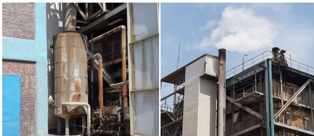
Fig. 5. Image of blowdown tank, blowdown outlet towards the outlet channel and blowdown vapors in Loshan power plant
