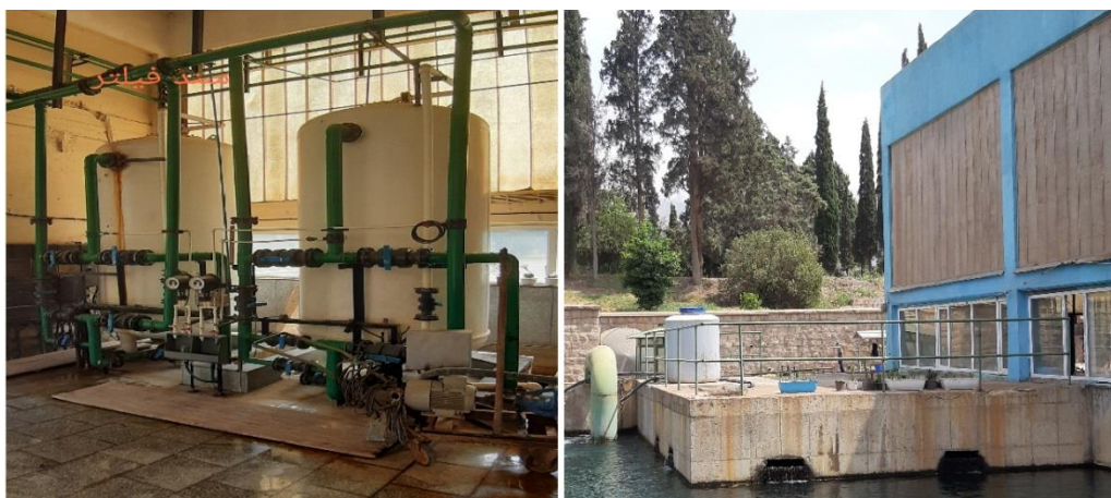
Fig. 3. The image of the sand filters and the produced water stored in the closed pond after passing through the sand filters
