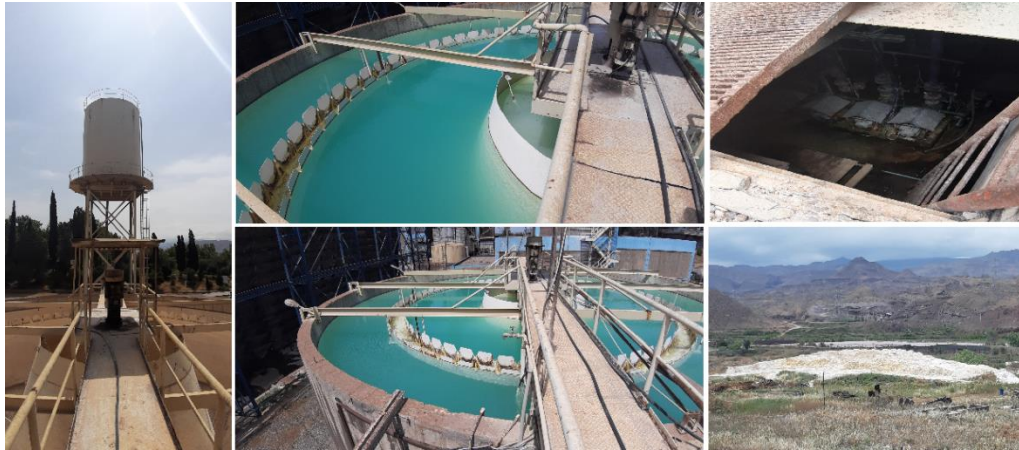
Fig. 1. Image of the air storage source, clarifier, sludge and wastewater transfer pumps, and the storage place for sludge and clarifier sediments
