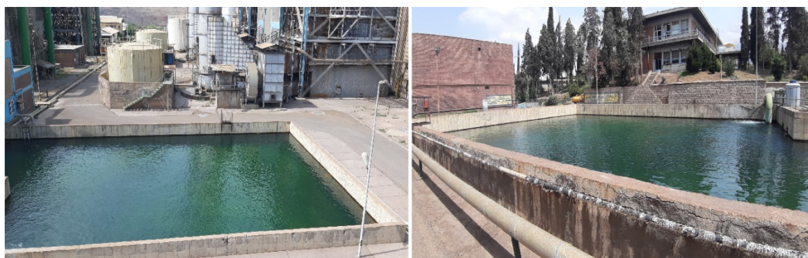
Fig. 2. Picture of the open pond of Loshan power plant
