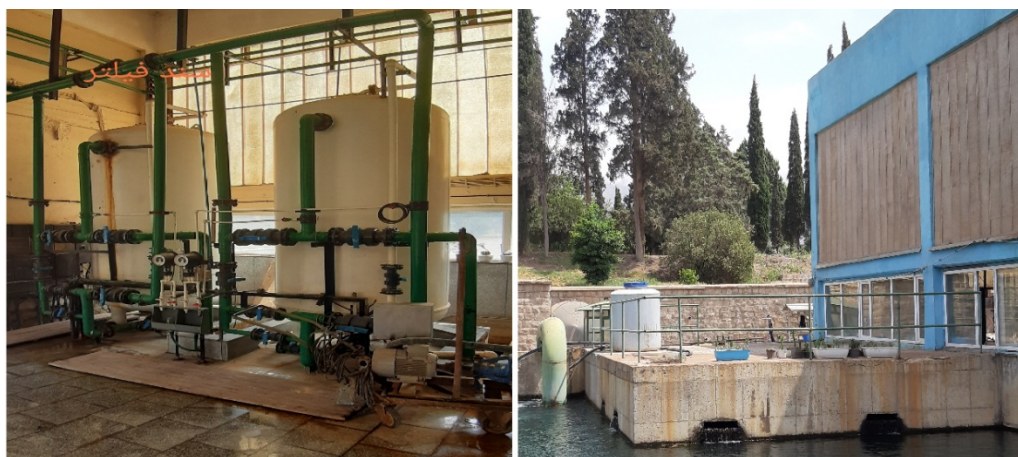
Fig. 3. The image of the sand filters and the produced water stored in the closed pond after passing through the sand filters
