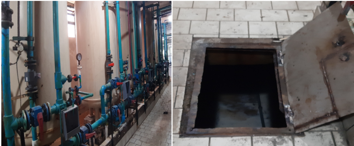
Fig. 4. The image of cationic, anionic and mixed-bed filters and the neutralization pond of resin regeneration effluents
