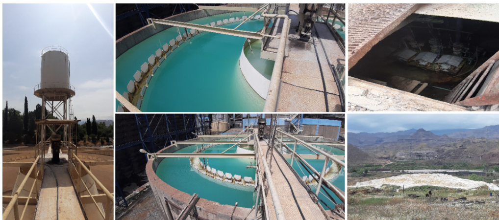
Fig. 1. Image of the elevated water storage tank, clarifier, sludge and wastewater transfer pumps, and the storage place for sludge and clarifier sediments
