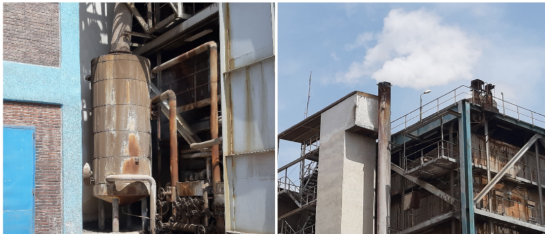
Fig. 5. Image of blowdown tank, blowdown outlet towards the outlet channel and blowdown vapors in Loshan power plant
