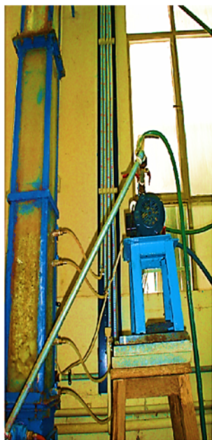
Fig. 1. Actual image of the filtration system employed in this study
