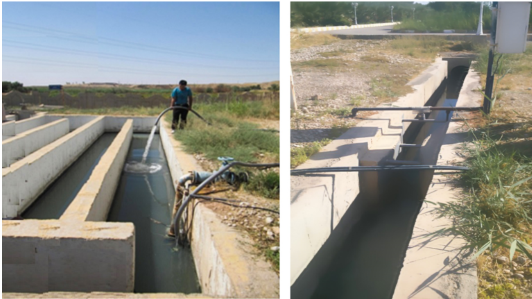
Fig. 3. Pumps, pipes and fittings to completely direct the treatment plant effluent to the pool
