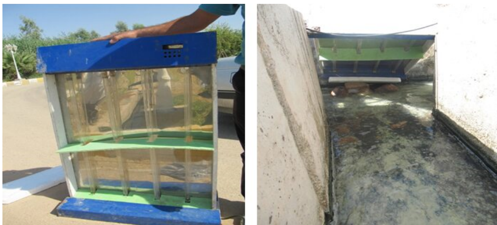
Fig. 5. Installation of UV lamps before the effluent enters the fish pond
