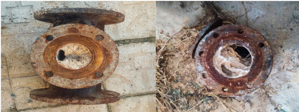
Fig. 9. Sedimentation formed on water distribution network components
